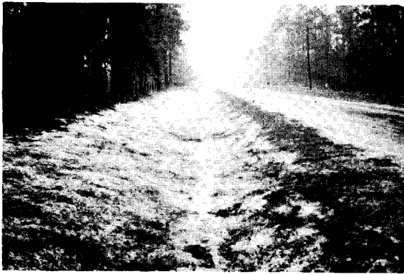
Figure B-3 Test Channel No. 1-FGR lined with fiber glass roving and asphalt tack. A light rain had just stopped.
