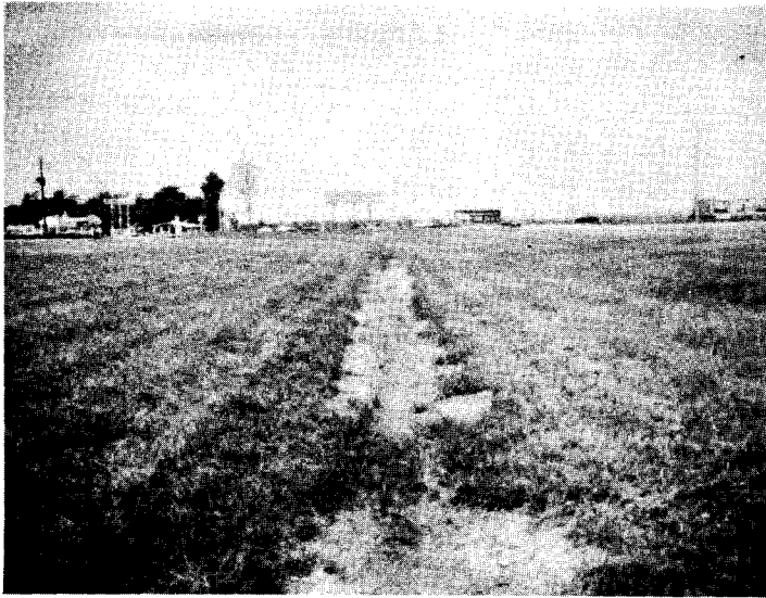
Figure 23. Asphalt Cement and Fiber Glass Roving Liner Over Sterilized Soil After Two Years
