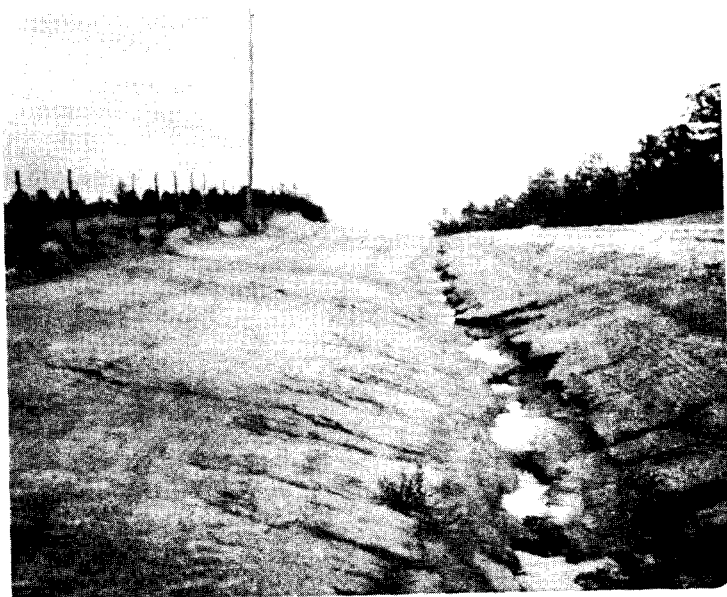
Figure 11. Typical Erosion Damage to Newly Seeded Channel
